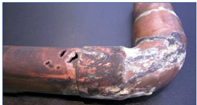
Figure 2. Pinhole leaks in copper tubing caused by internal corrosion.
