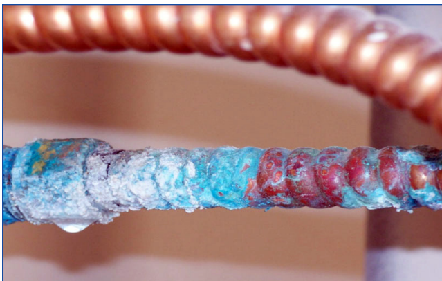
Figure 1. Corrosion at a connection on a water heater indicated by the blue-green color.
